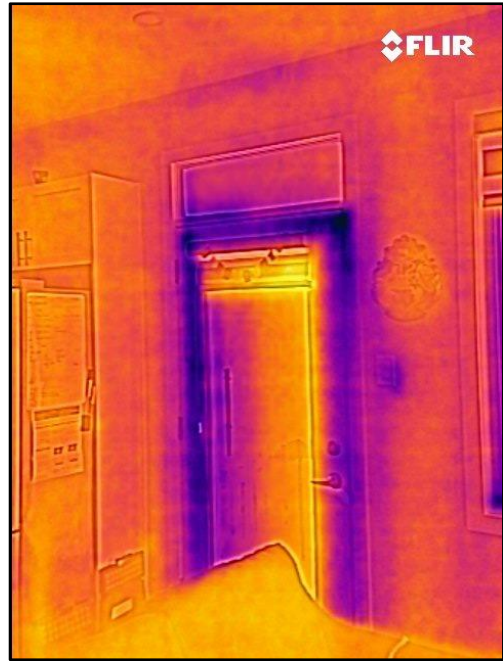
74. 8.2 Air infiltration through windows and...
