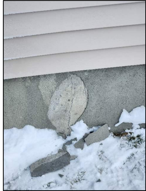
59. 1.8 Parging (not brush coating) is falli
