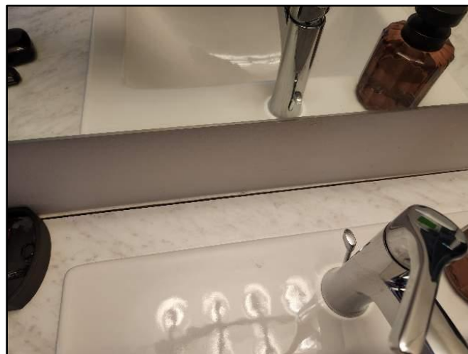
37. Caulking missing or ineffective
