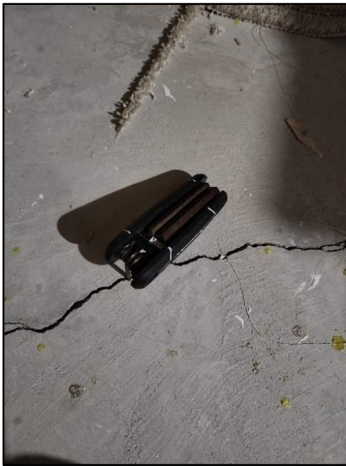
56. 1.4 Concrete basement floor is cracked.
