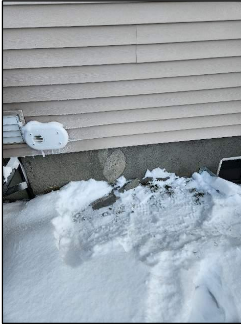
58. 1.8 Parging (not brush coating) is falli
