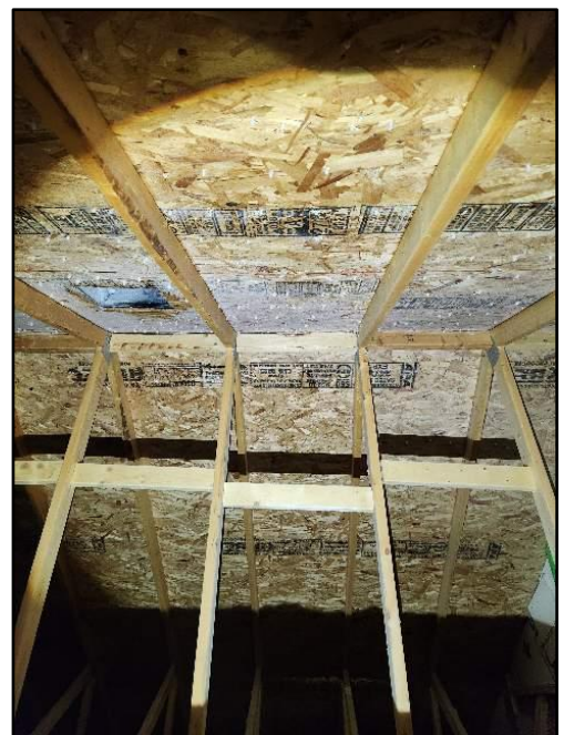
66. 5.0 Missing, Incomplete or Damaged Items
