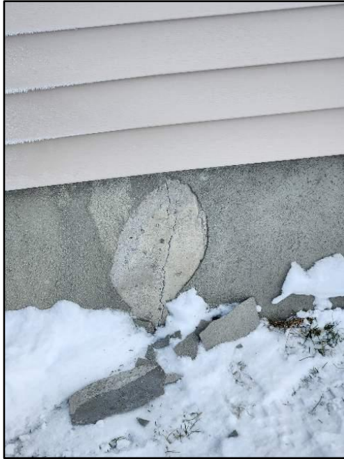
14. Typical minor cracks
