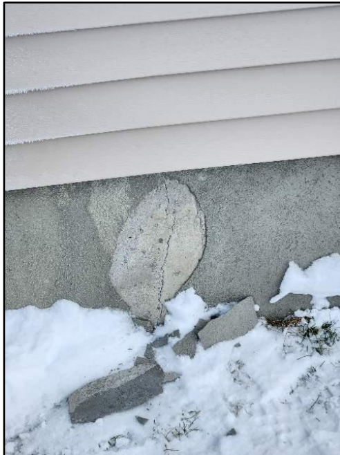
16. Parging damaged or missing
