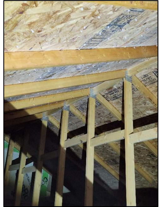
68. 5.0 Missing, Incomplete or Damaged Items
