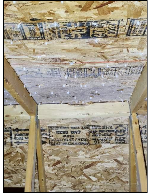
64. 5.0 Missing, Incomplete or Damaged Items
