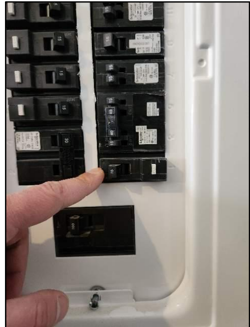
25. Loose breakers or fuses
