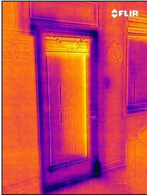
77. 8.2 Air infiltration through windows and...
