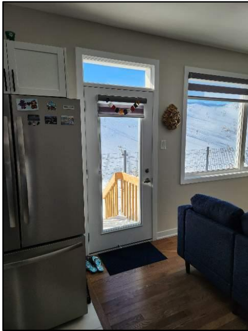
73. 8.2 Air infiltration through windows and
