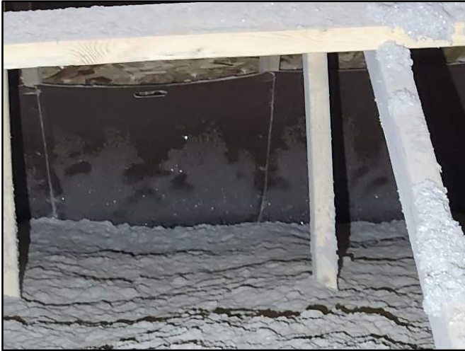
67. 5.0 Missing, Incomplete or Damaged Items
