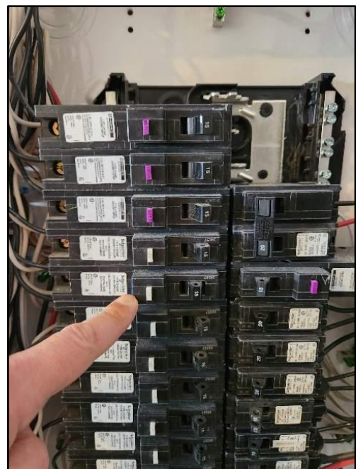
72. 7.1 Fuses blow or circuit breakers trip.
