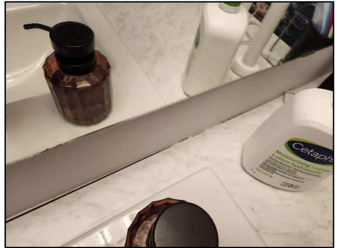
36. Caulking missing or ineffective
