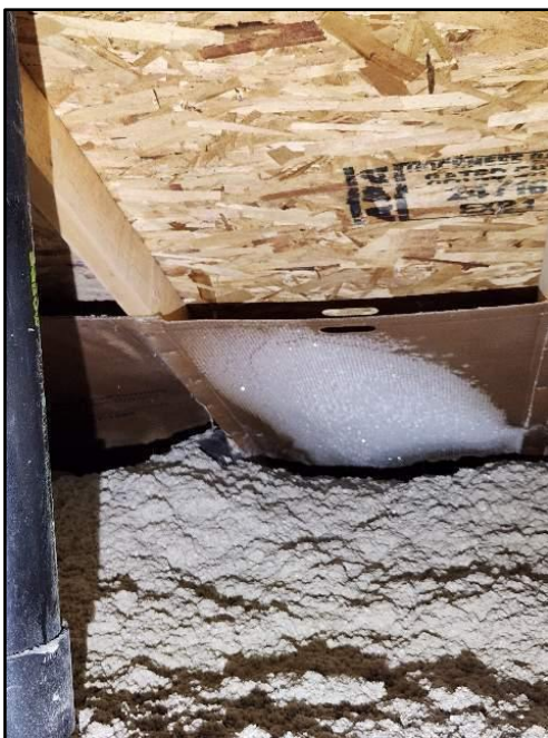
65. 5.0 Missing, Incomplete or Damaged Items
