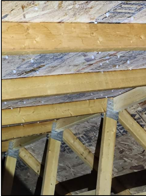
63. 5.0 Missing, Incomplete or Damaged Items
