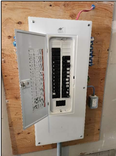
24. Loose breakers or fuses
