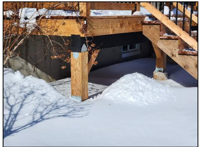
29. Parging damaged or missing
