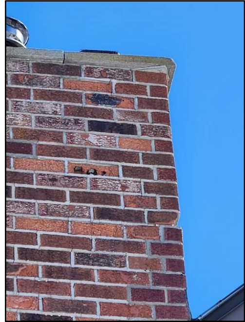
52. Loose, missing or deteriorated masonry
