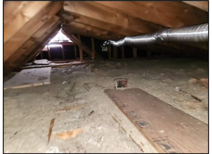
65. Amount less than current standards
