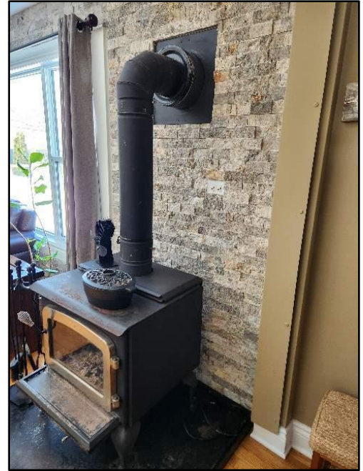
62. Firebrick cracked, crumbling or incomplete
