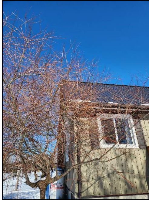
1. Tree branches touching roof
