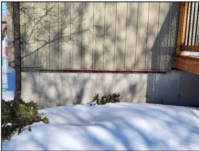
28. Parging damaged or missing
