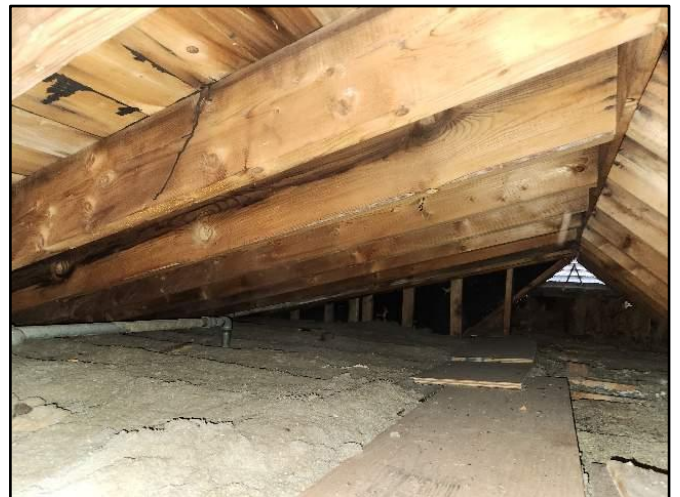
67. Amount less than current standards
