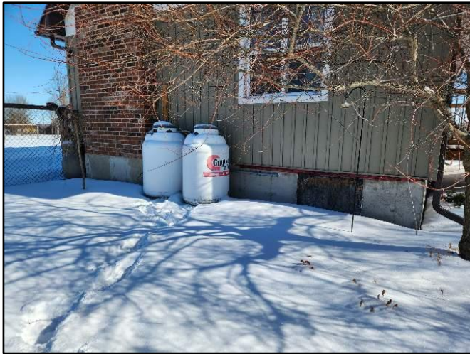
26. Parging damaged or missing
