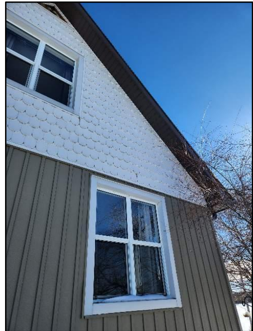
15. Loose or missing pieces
