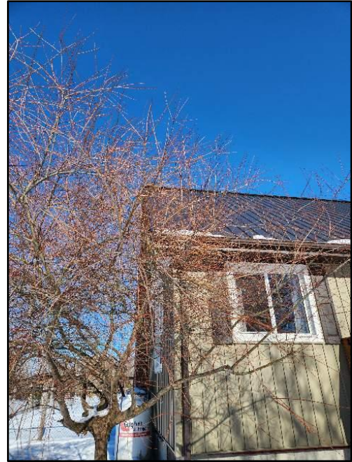
22. Trees or shrubs too close to building
