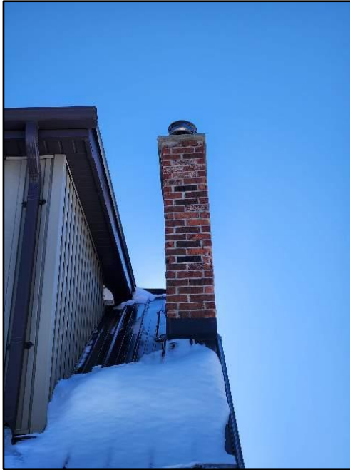
53. Settling or leaning
