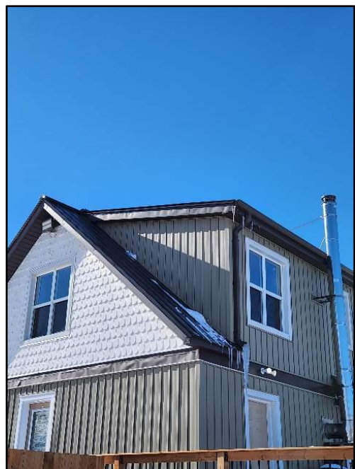
7. Siding not cut back
