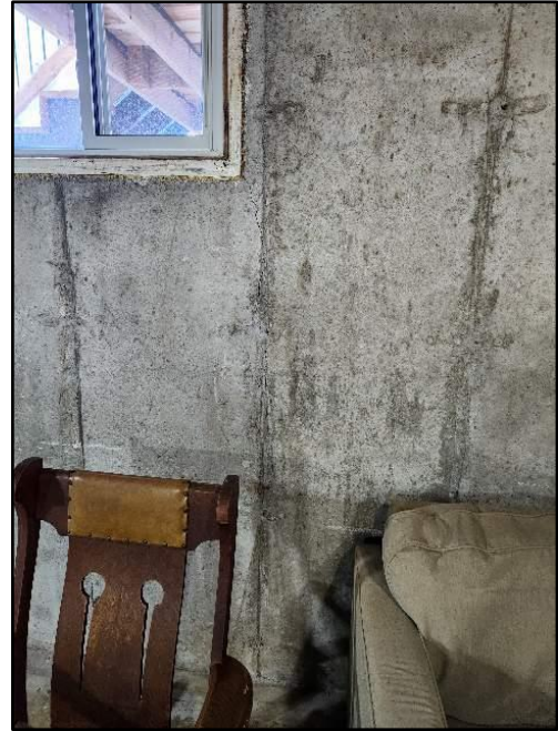
25. Typical minor cracks
