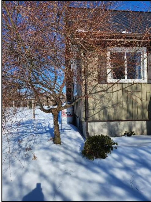
21. Trees or shrubs too close to building
