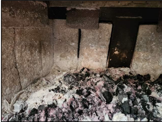
61. Firebrick cracked, crumbling or incomplete
