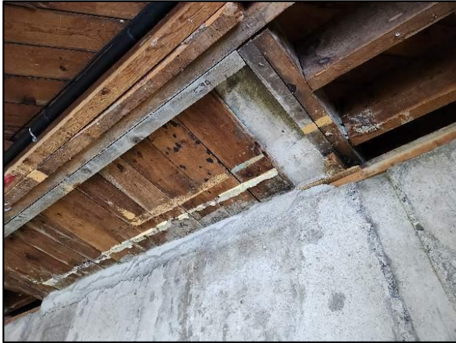
55. Wood forms not removed
