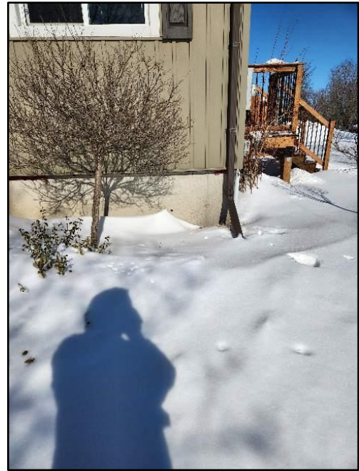
31. Parging damaged or missing
