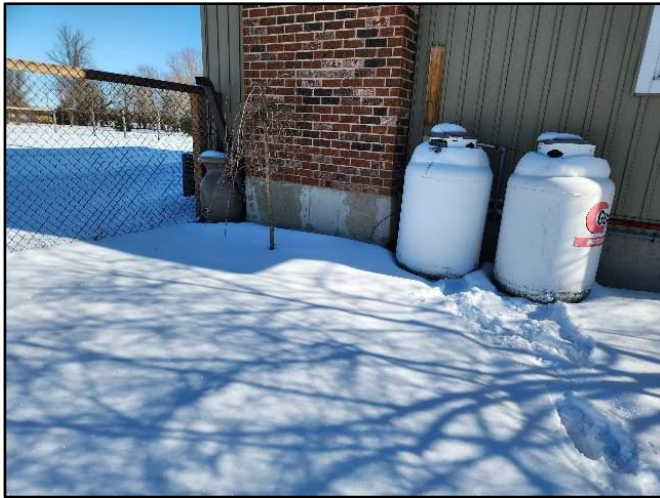
30. Parging damaged or missing
