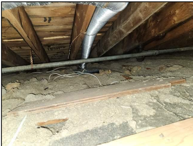
66. Amount less than current standards
