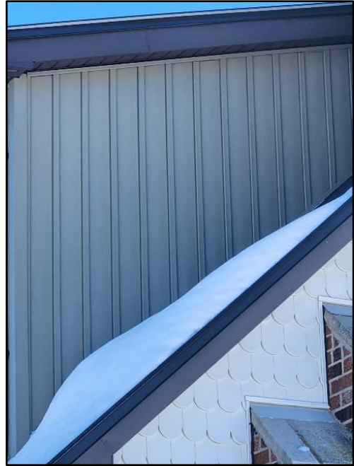
5. Siding not cut back
