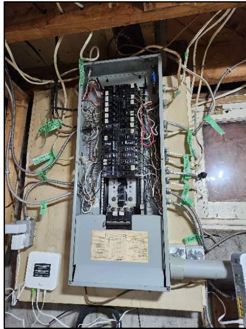
42. Loose breakers or fuses
