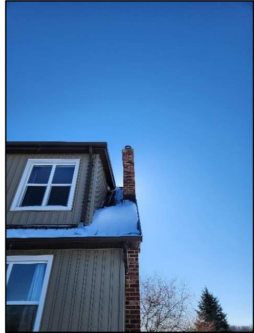
54. Settling or leaning
