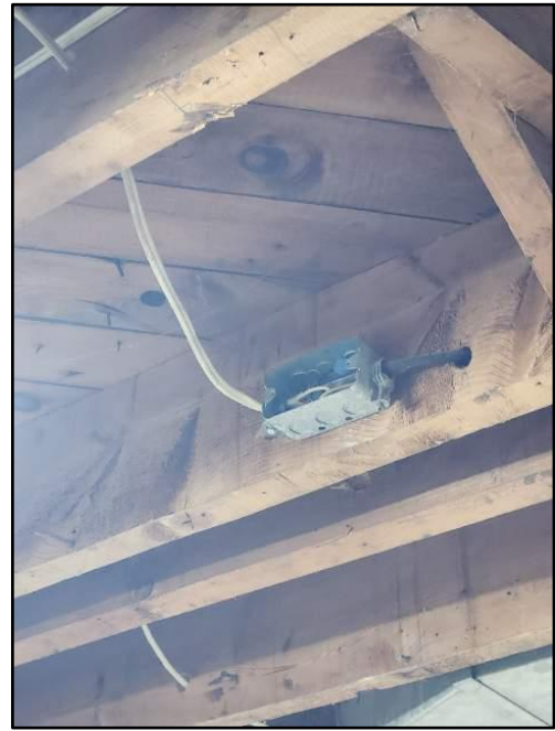
48. For junction box is missing
