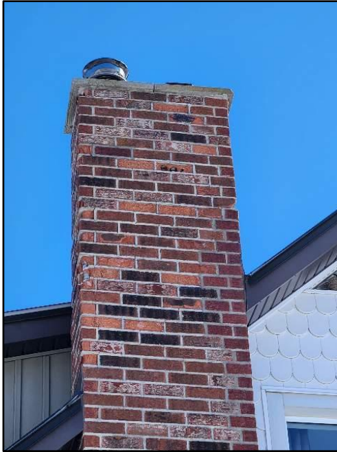
51. Loose, missing or deteriorated masonry
