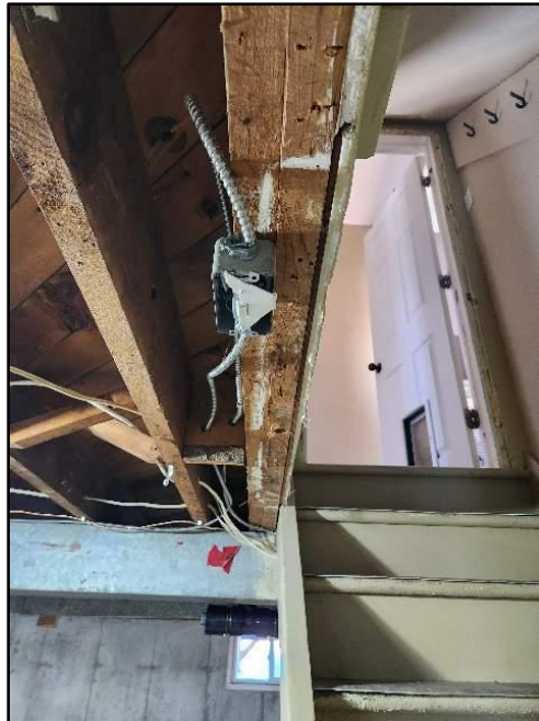
46. For switch is damaged
