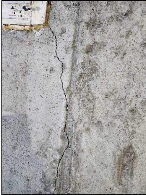
24. Typical minor cracks
