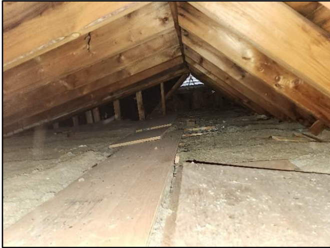
64. Amount less than current standards
