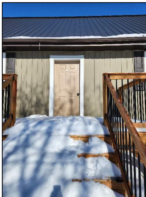
20. No step up into building
