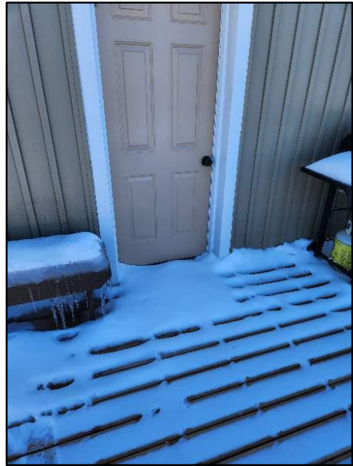
19. No step up into building
