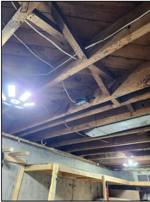
47. For junction box is missing
