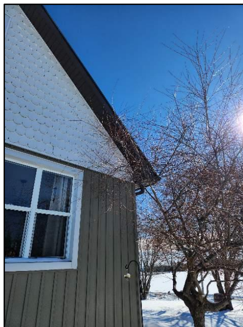
23. Trees or shrubs too close to building
