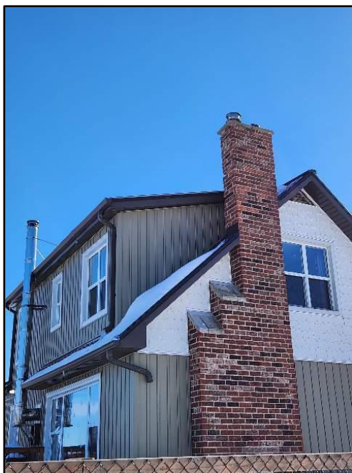
6. Siding not cut back
