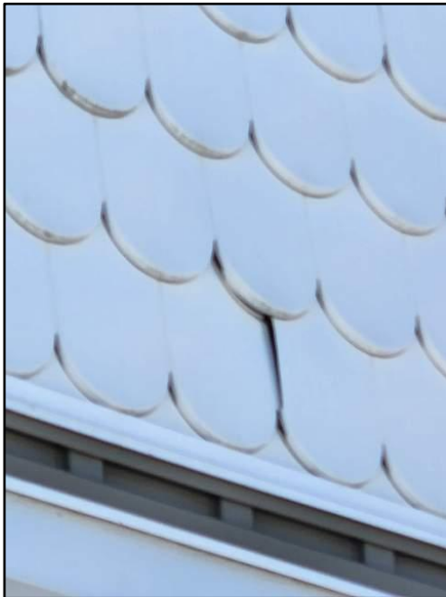
14. Loose or missing pieces
