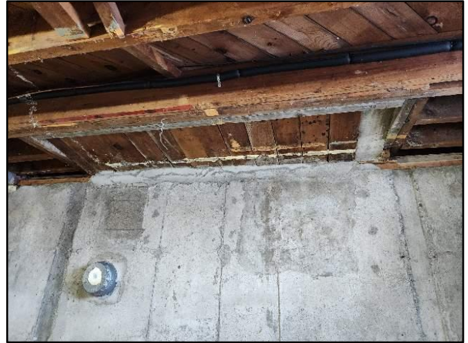
56. Wood forms not removed
