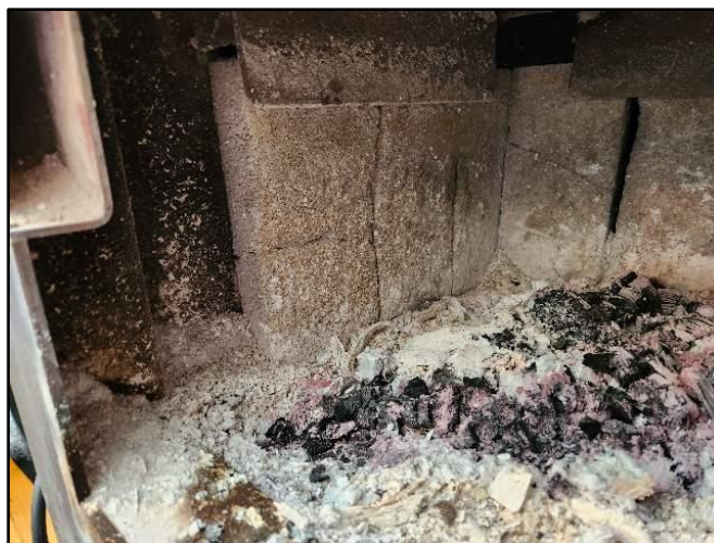
63. Firebrick cracked, crumbling or incomplete
