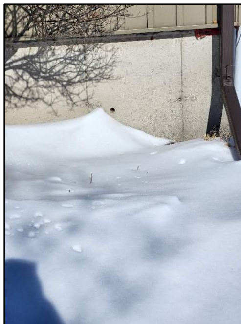
32. Parging damaged or missing
