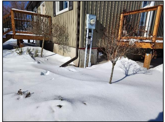
27. Parging damaged or missing
