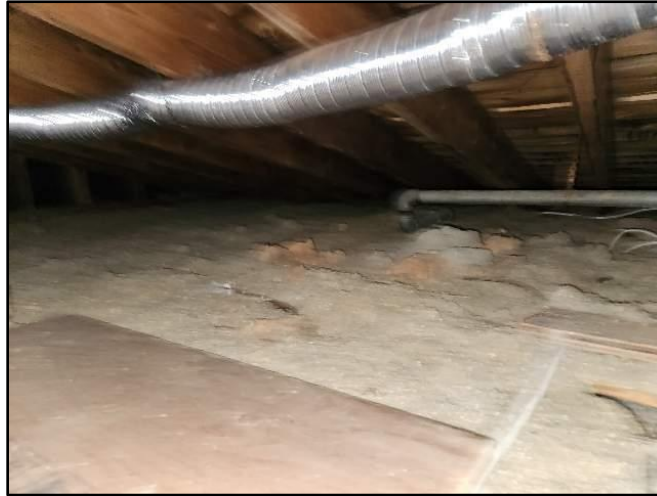
68. Amount less than current standards
